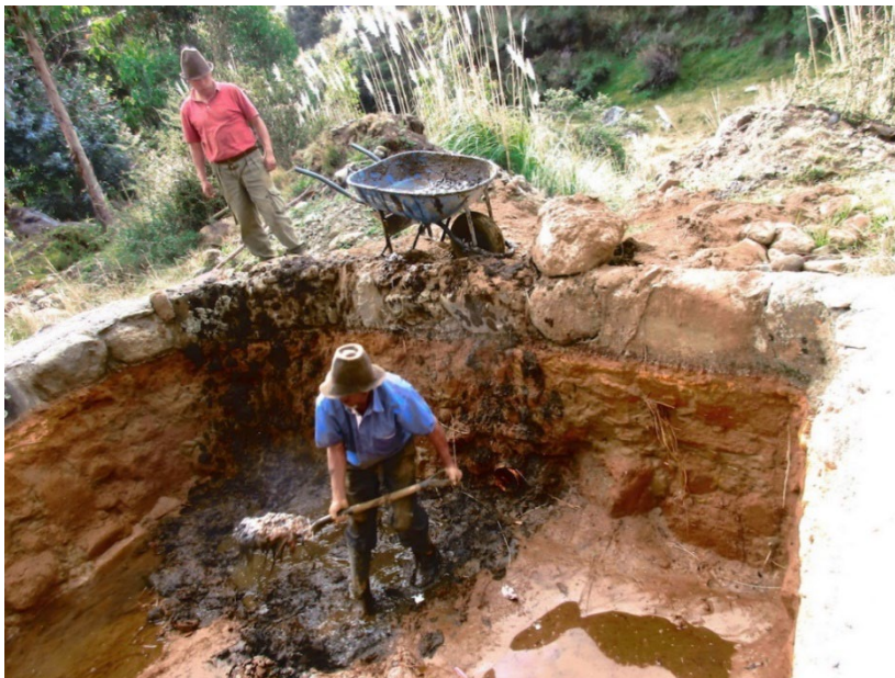
Figure 2. Cleaning of sedimentation ponds (Image sourced from Panorama case study (Doris Chavez), © Mountain Institute).
